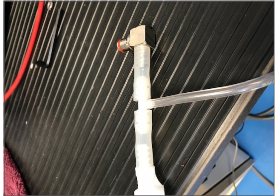
View of the alarm connection.
